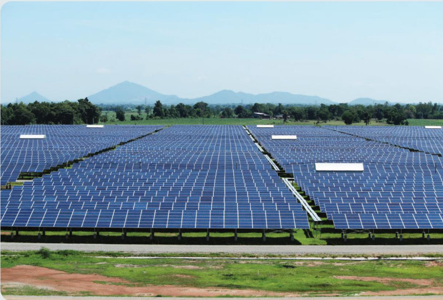
▲ A solar farm
